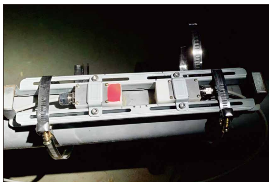
Copper industry – tap water pipe
