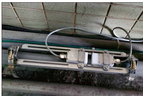
Food industry – pure water boiler pipe
