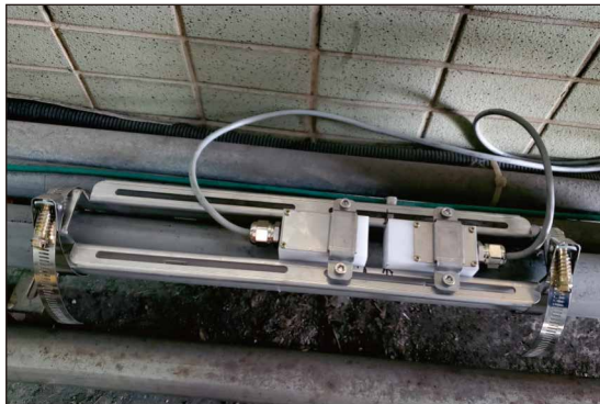
Food industry – pure water boiler pipe
