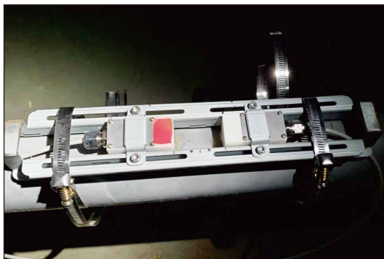
Copper industry – tap water pipe
