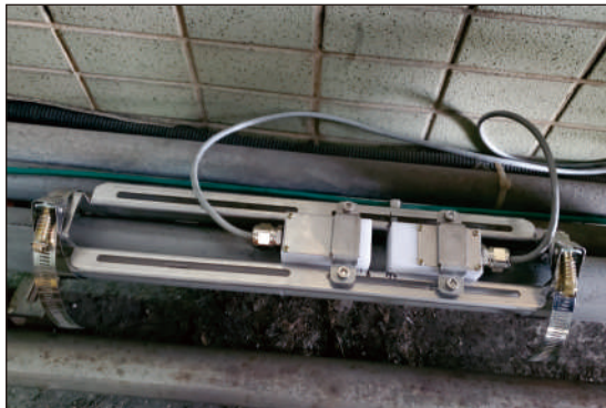
Food industry – pure water boiler pipe
