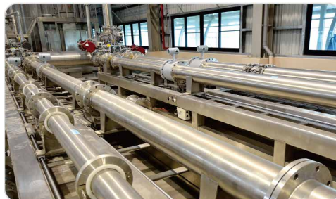
Piping system II (Maximum diameter is 500mm)
