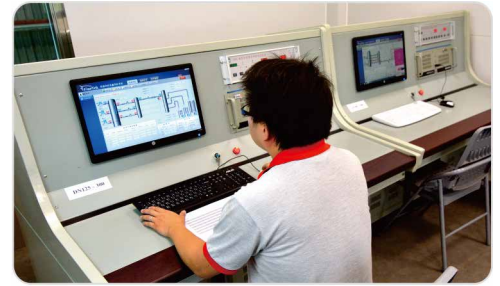
Control room & Graphical HMI
