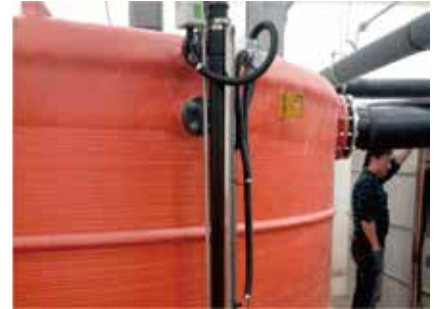
Cooling water reserve detection of electronic plants
