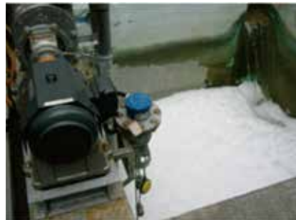
Wastewater level detection
