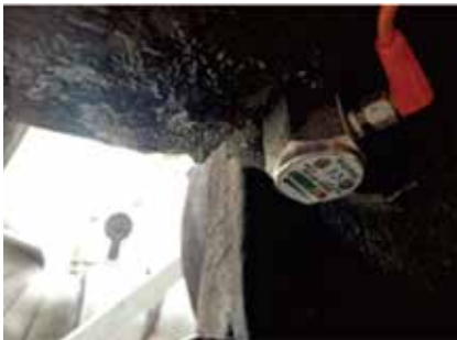
Pipeline flow detection
