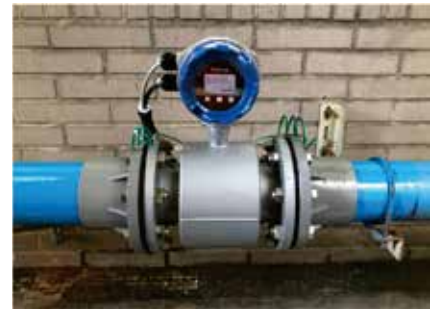
Wastewater flow detection
